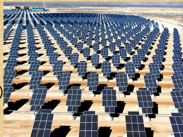
70,000 solar panels, generates 14 MW of solar power, Nevada, United States
